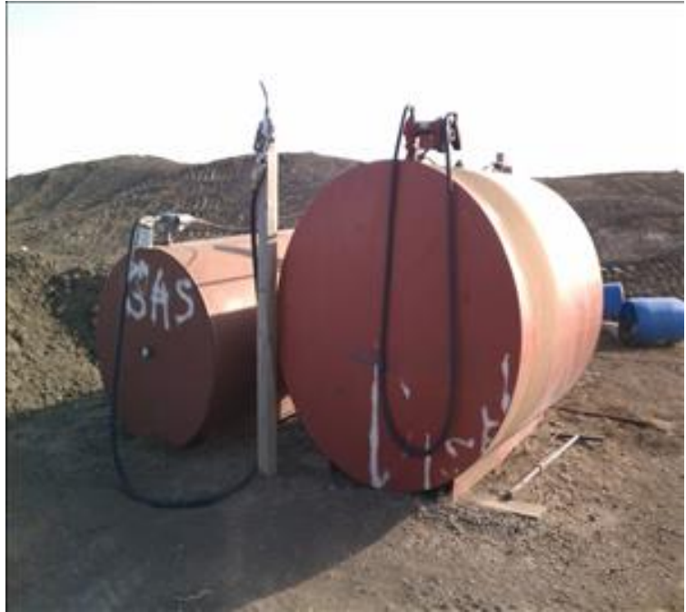
No labels and no berm.
